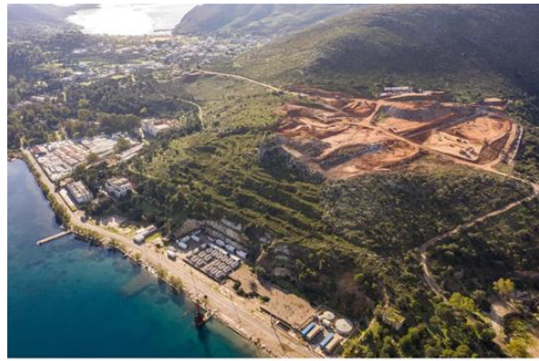
The construction site of the Leros camp seen from the sky in March 2021. Since then, rows of containers have been installed on the site to accommodate the migrants.
